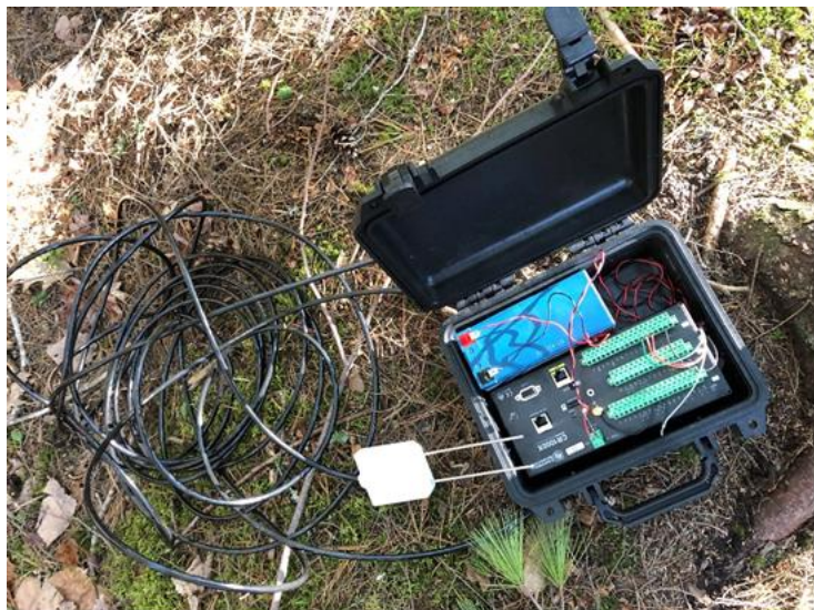
Soil moisture sensors and data acquisition system at Old Town site.
