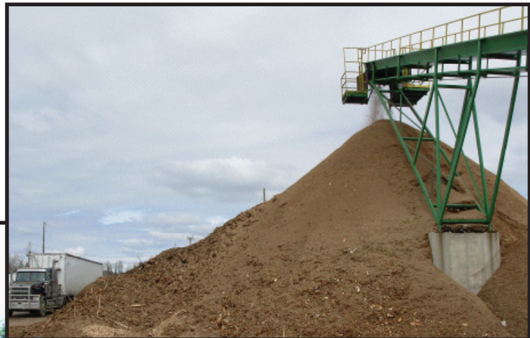
Wood to electricity: chip pile for electric plant.
